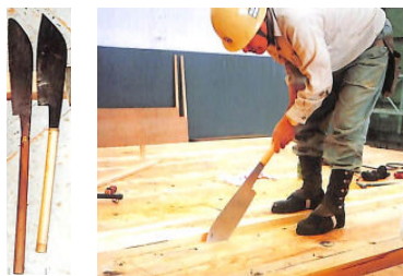
Fig.10 'Surinoko' saws for preparing the surface of plates to mate each other to keep water tightness
