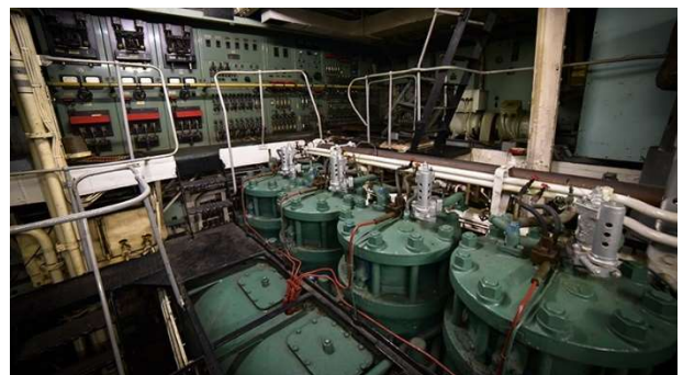
Fig.9 Engine Room of Soya
